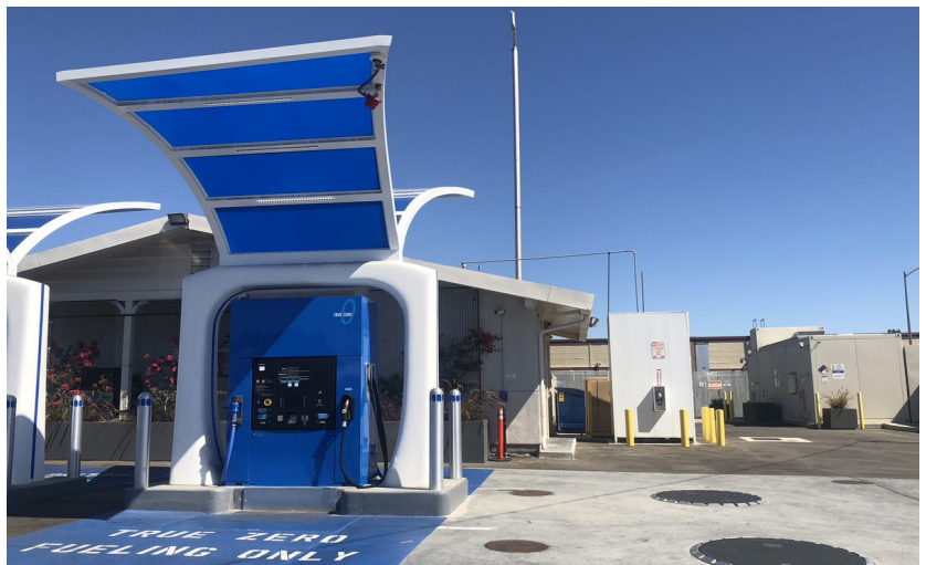
Hydrogen Fueling Station - Vacuum Insulated Cooling Lines
