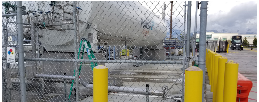
Hydrogen Extended Fill Line
