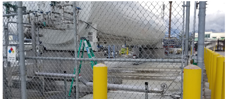
LH2 Vacuum Insulated Pipe and Extended Trailer Fill Lines
